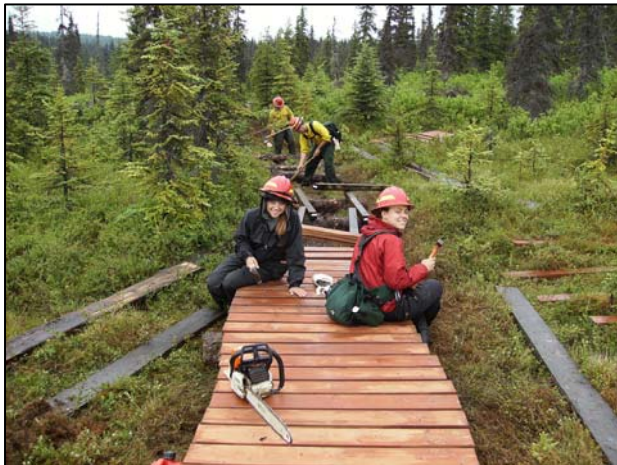
Trail crew, working on the installation of boardwalk in the Homer Demonstration Forest. This project was completed in the summer of 2007.
