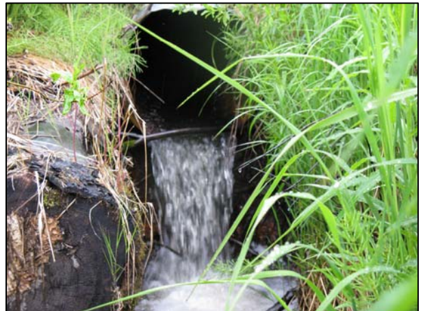
Santiago Lane, Northeast of Anchor Point, This 24 inch perched culvert creates a barrier to juvenile salmon. The Homer District has the plans completed to replace this during the summer of 2008.
