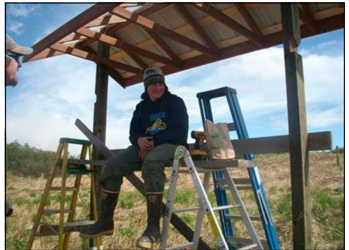
Jake McLean takes a bit of a rest during the installation of his kiosk in the Snomads parking lot at the trailhead of the Watermelon Trail. Jake organized a sizable work party to install this mammoth informational kiosk
