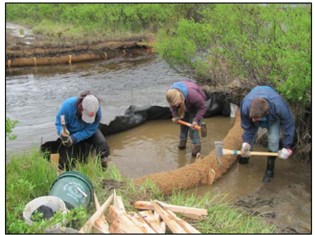
Members of the Youth Conservation Corps placing coir logs along the damaged banks. Coir logs are used for erosion control in areas of low wave energy. Overtime they will disintegrate, leaving the bank completely restored. Note the opposite bank compared to the top photo, installation is completed on that side.
